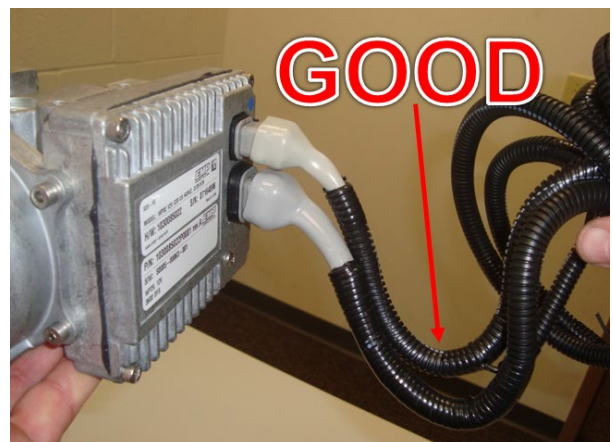
Good Wiring – Drip loops
