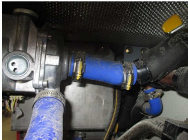
Improper installation with localized high spots
